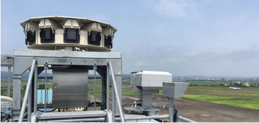
Fig. 2 OTW cameras and PTZ camera system at Sendai airport
