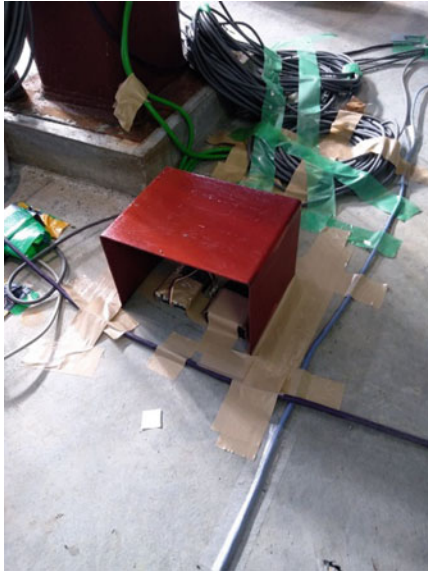
(a) Sensor unit on first floor
