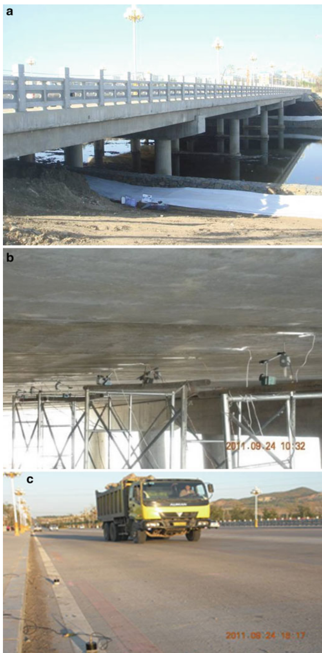
Fig. 2 Field test: a appearance of the bridge; b displacement sensors layout; c acceleration sensors layout
