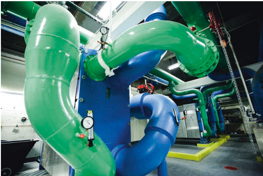
Fig. 4.9 DEN CUP piping. (Courtesy of Denver International Airport)
