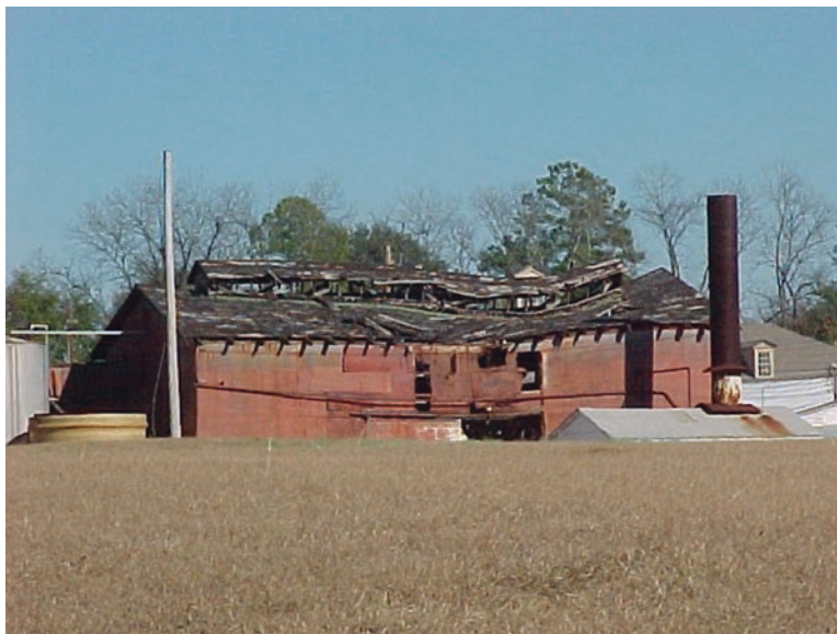
Fig. 15.10 Some of the buildings were in poor condition and required demolition. Special handling during demolition and disposal was required for some buildings with contaminated building materials
