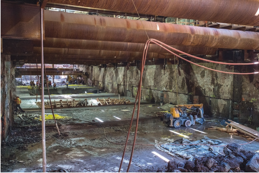
Fig. 12.14 NYC MTA’s Second Avenue Subway cut and cover construction of 96th Street Station. (Source: cc. Metropolitan Transportation Authority/Patrick Cashin)
