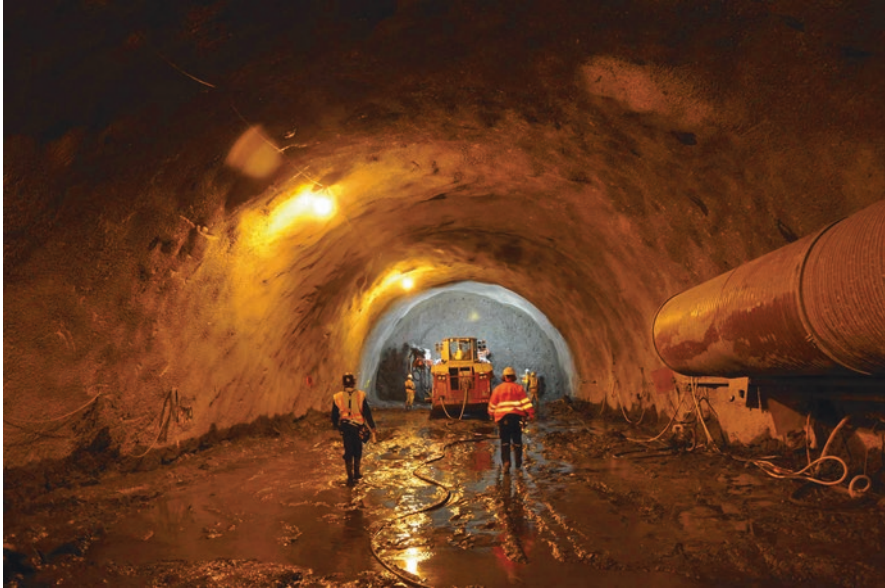
Fig. 12.17 SEM excavation on the Devil's Slide Tunnel, in California. (Source: Tunnelling Journal)
