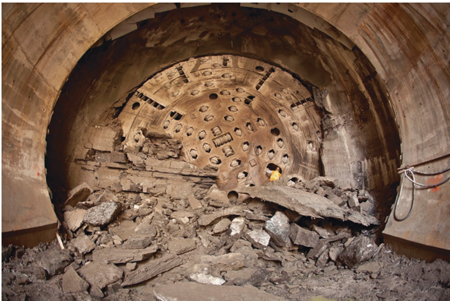
Fig. 12.9 A 47.5-ft-diameter Robbins TBM “breaks through” on the Niagara Tunnel Project, in Canada, in 2011. At the time, it was the world’s largest rock TBM. (Source: Robbins)
