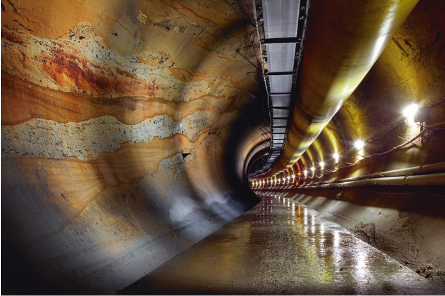
Fig. 12.15 Unlined rock tunnel on the Epping to Chatswood rail link, in Sydney, Australia. The tunnels were excavated by two 23.6 ft-diameter Robbins Main Beam TBMs. (Source: Robbins)
