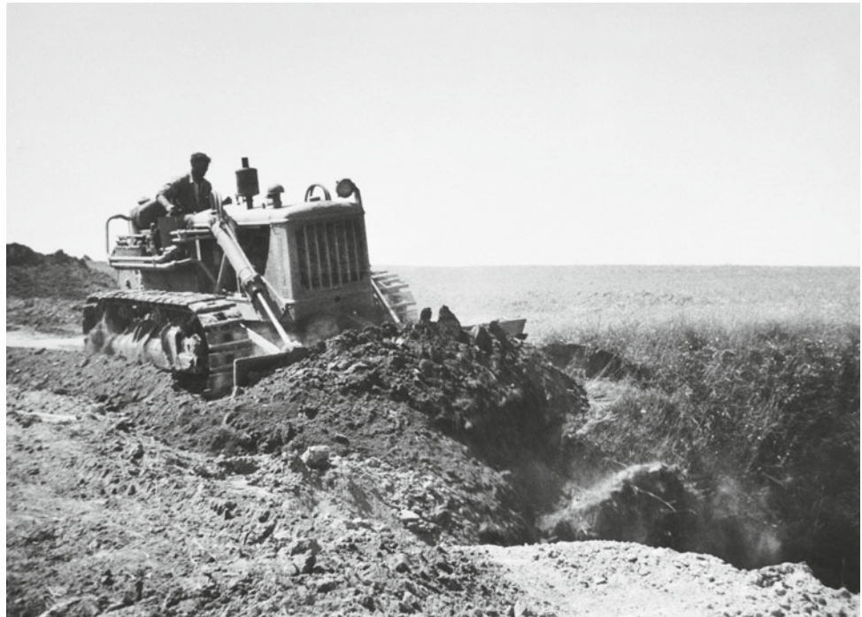
Fig. 11.6 Filling of a sunken road in 1949 in Hippersdorf (close to Königsbrunn am Wagram as located in Fig. 11.3) to increase parcel size and prevent further gully erosion. Source Abt. Güterwege, Provincial Government of Lower Austria
