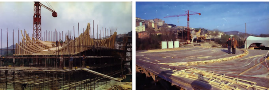
Fig. 20 Bridge over the Basento river in Potenza, 1967–1975, S. Musmeci: the complex construction site. Courtesy Edilstrade Archive (SIXXIdata)
