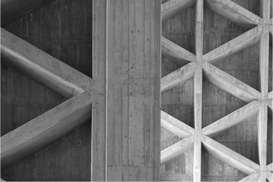
Fig. 8 The roofing of the Marian Temple, Trieste, 1963–1967, S. Musmeci, A. Guacci. Photo Sergio Poretti (SIXXIdata)
