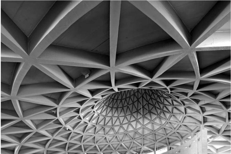
Fig. 6 The roofing of the San Carlo Church, Villaggio del Sole, Vicenza, S. Musmeci, S. Ortolani, 1960–1962. Photo Sergio Poretti (SIXXIdata)
