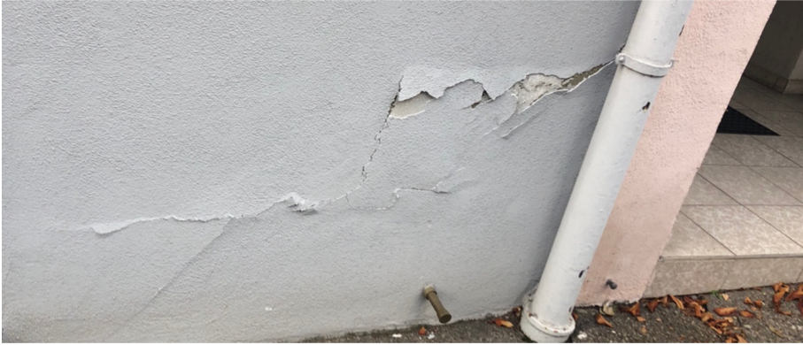
Fig. 6. Cracks in the building started to appear at the same time (May 2019) as the observed release rupture in the time series (Fig. 5).
