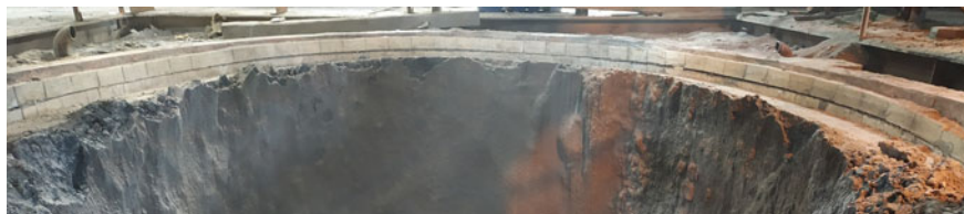
Fig. 4 Lead ISASMELT™ furnace side wall bricks, exposed mid-campaign, showing widespread spinel coating
