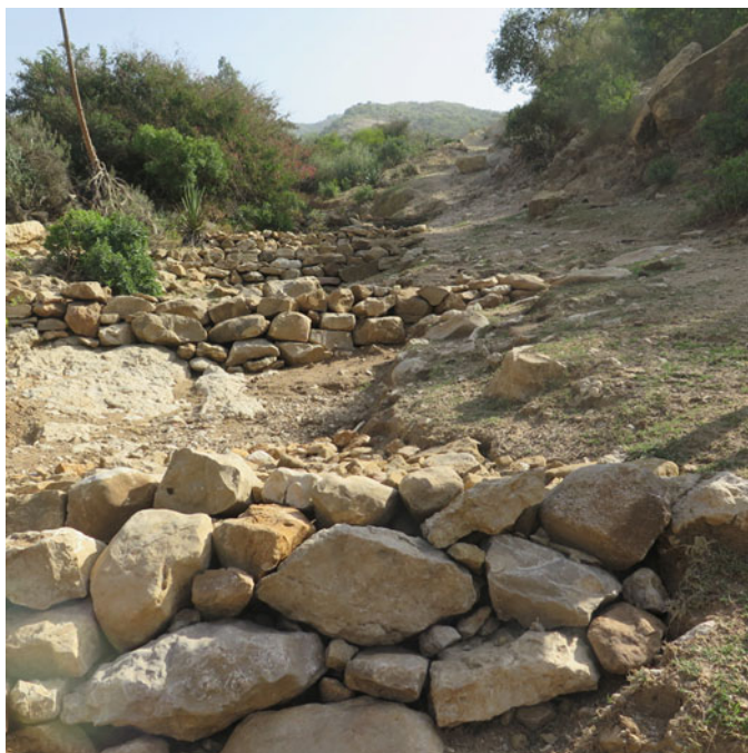
Fig. 26.3 Newly constructed check dams in an outwash area in Abreha we Atsbeha. (Photo: E. Sigman)
