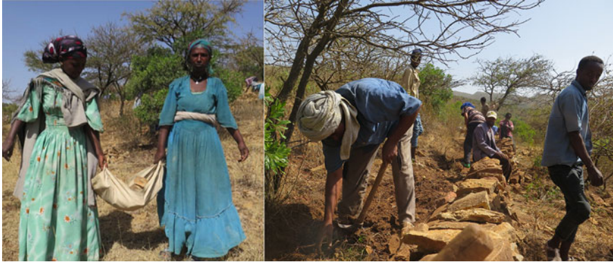
Fig. 26.1 Free Labour Contribution Period (FLCP) activities. On left: two women use a repurposed food sack to carry stones from the excavation site to the terracing site. On right: A mixed group of men and women construct a stone terrace. These activities happen side by side continuously. (Photos: E. Sigman, with permission from community members photographed)
