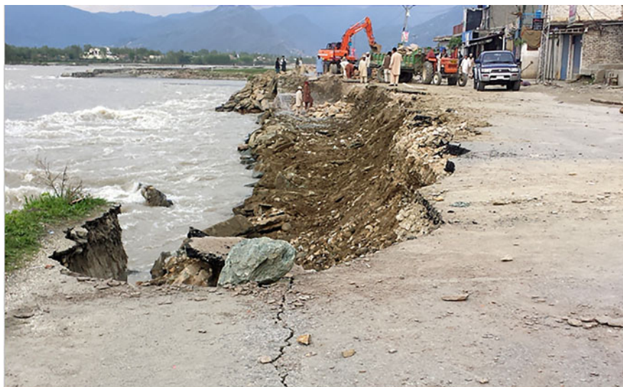
Fig. 11.2 Roads and highways are destroyed as a result of floods
