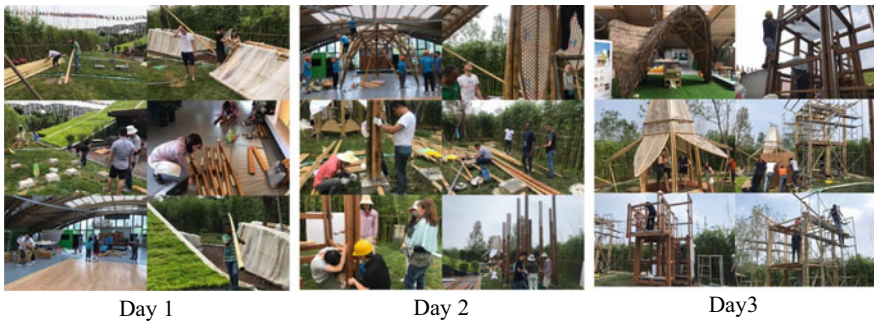
Fig. 5 Some photos of the three days of construction at the 2019 Beijing Horticultural Expo to build the proposed design project from July 17th to July 19th, 2019
