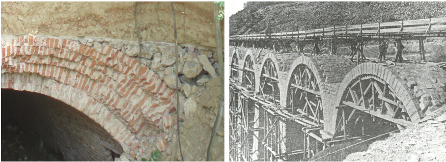
Fig. 2. Left: Stone backing of brickwork arch (bridge under demolition, Hungary), Right: Haunching between piers (bridge under construction, Hungary)
