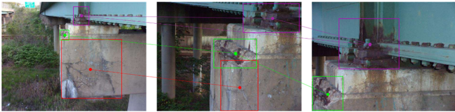
Fig. 1. Defect matching example. Different defect types are drawn in different colors. Defect matching is performed between all relevant image pairs. Multiple instances of the same defect were correctly matched across different drone images. Green bounding box: exposed reinforcement defect correctly detected across multiple images. Defect matching is represented by the lines between different occurrences of a specific defect.
