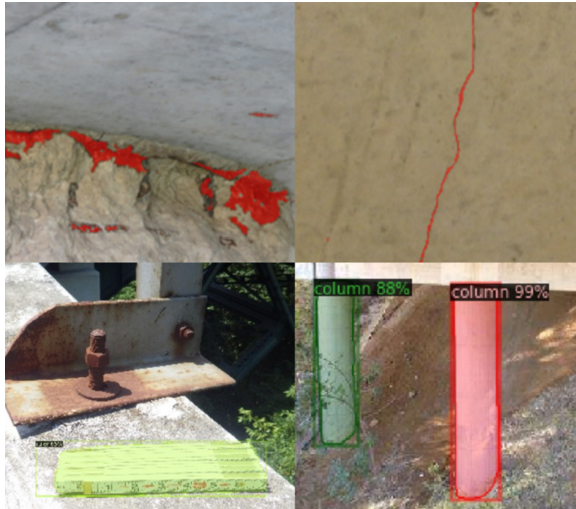
Fig. 3. Top row: semantic segmentation of corrosion (left) and cracks (right). Bottom row: instance segmentation of rulers (left) and columns (right).
