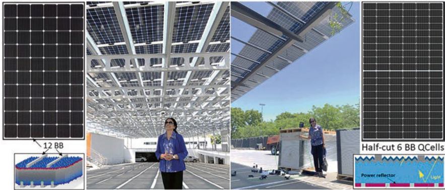
Fig. 7 Bifacial horizontal roof top solar arrays using 12 multi-busbar mono-Si modules (left); inclined half-cut 6 busbar Q-cells panels (right) under installation at Bishop Ranch, California. Single panel and cell schematics are shown. (Photo courtesy Distributed Solar Development)
