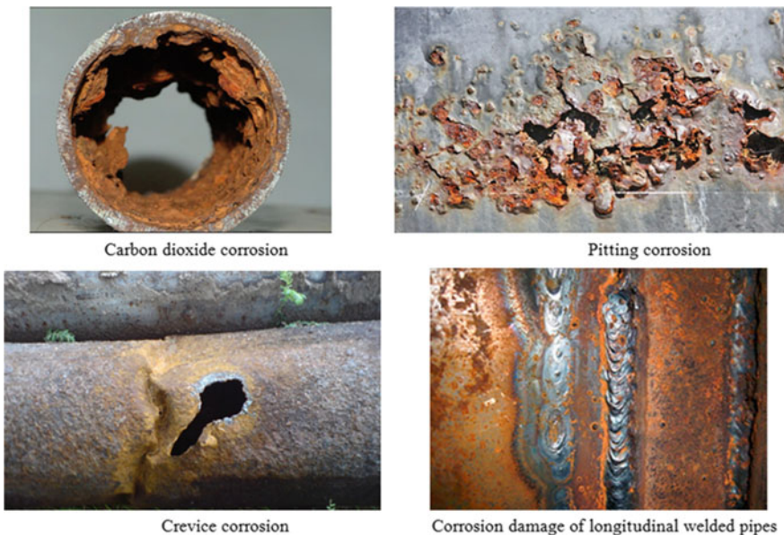
Fig. 1 Corrosion variants of thermal network steel pipelines
