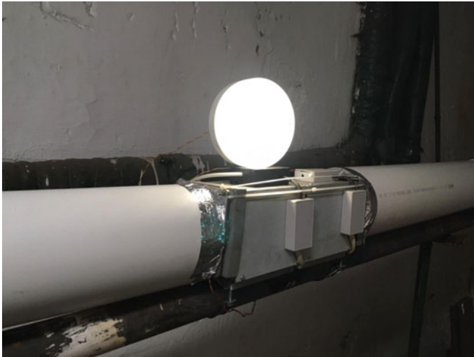
Fig. 4 Thermoelectric generator for the sewerage system
