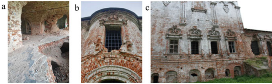
Fig. 3 a Condition of internal structures; b condition of decoration and openings of the altar part; c condition of the north facade
