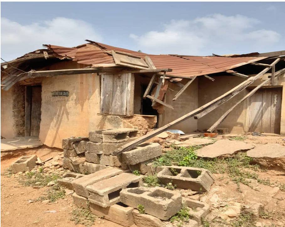
Fig. 1. An example of a building in Nigeria where some people are living. Source: The researcher, March 26, 2021
