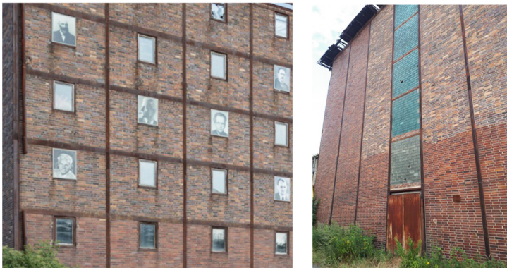
Fig. 9. Outer steel skeleton with corrosion damage
