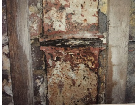
Fig. 10. Column in the building with corrosion damage
