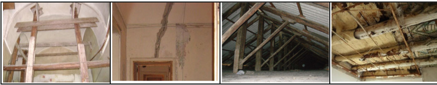
Fig. 2. Typical damage in masonry and wooden structures.
