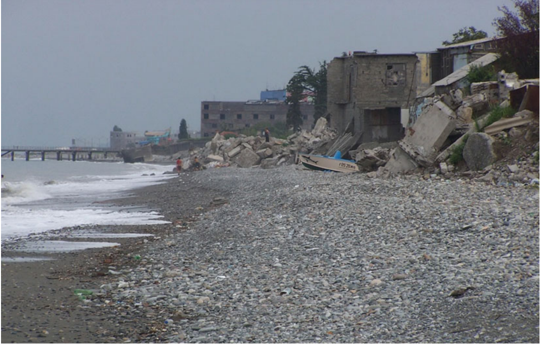
Fig. 9.2 The emergency section on the southern periphery of the Batumi city coast 2005 (photo by G. Lominadze)
