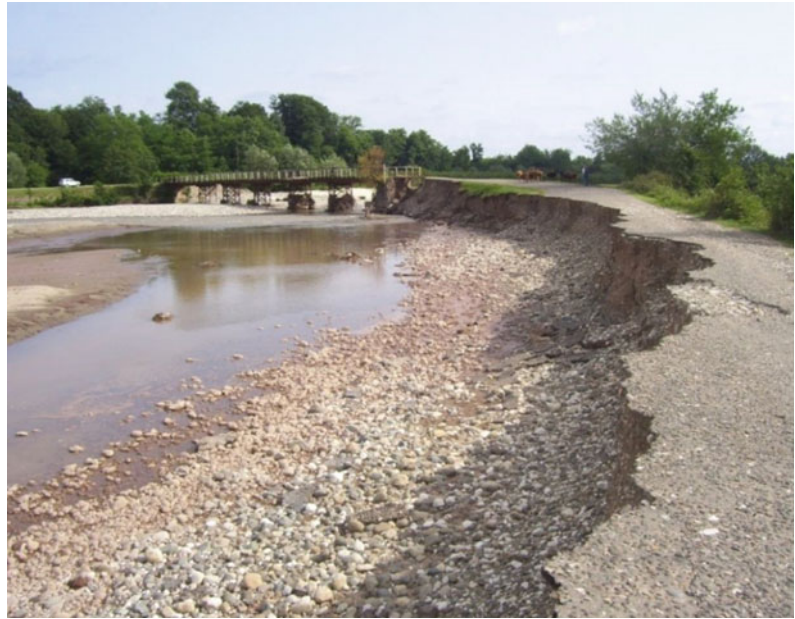
Fig. 7.11 River Bank erosion in Khobi Municipality, 2009 (photo by G. Gaprindashvili)
