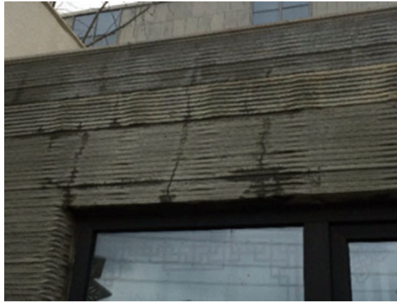
Fig. 5.14 Early age shrinkage cracking in 3D printed walls (Schröfl et al. 2019)
