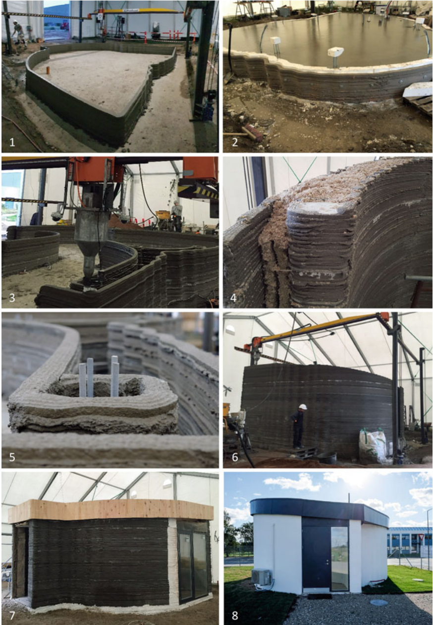
Fig. 2.11 Main phases in the construction of the BOD: 1. 3DCP of the foundation slab contour; 2. Concrete casting of the foundation slab; 3. 3DCP of the building walls and printing nozzle; 4. Detail of the insulation material; 5. Detail of the manually added rebars; 6. The BOD walls right after printing; 7. Application of roof, doors and windows; 8. The BOD after its completion
