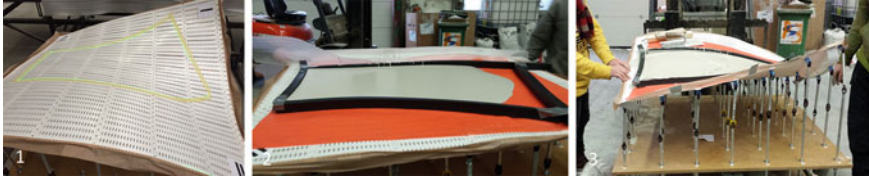
Fig. 2.20 Prototype of the flexible mould as developed in a Dutch R&D project operating in mode 1, deformation: Setting out formwork (Schipper et al. 2015b)
