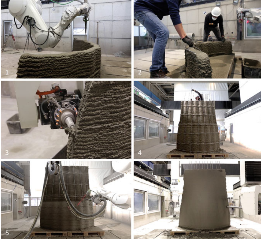
Fig. 2.12 Fabrication process; 1. Shotcrete 3D Printing of the wall; 2. manual placement of the pre-bent horizontal reinforcement; 3. precise cutting of the surface, while the concrete is still in the plastic state; 4. threading in the vertical reinforcement; 5. embedding the reinforcement by vertically spraying onto the printed structure; 6. final trowelling with a rotating plastic disc
