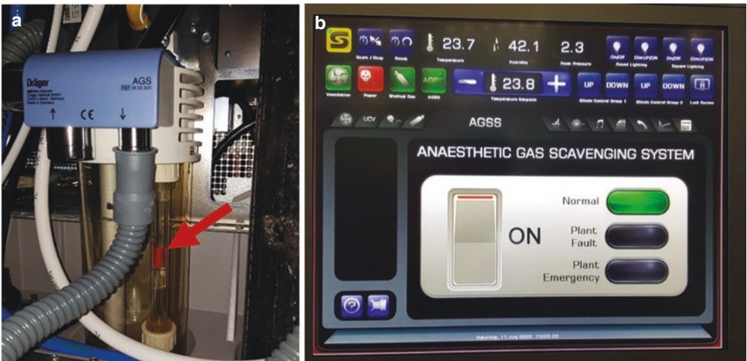
Fig. 5.11 Scavenging system. (a) Example of the scavenging interface within a Dräger anaesthesia machine. Red bobbin within adequate level (arrowed) (Dräger,
