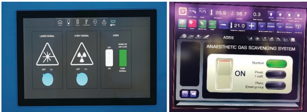
Fig. 10.1 Anesthesia gas scavenging system control panel
