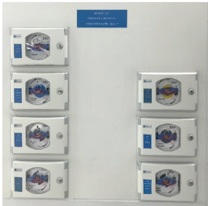
Fig. 10.6 Central gases control panel HMC-HGH
