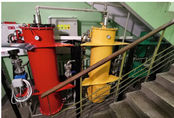
Fig. 17.3 Appearance of equipment for catalytic water purification with a gas-saturated reactor
