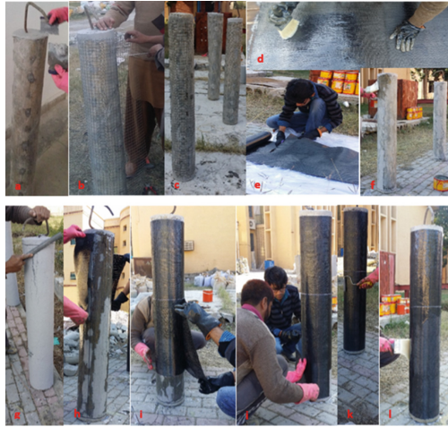
Fig. 2. a) Repairing of specimens, b) covering sample with steel wire mesh, c) sample wrapped with mesh, d) and e) Cutting and preparing CFRP, f) epoxy injected to samples, g) sample covered with cement sand mortar, h) and i) CFRP Wrap in progress, k) and L) sample repaired and ready for testing.
