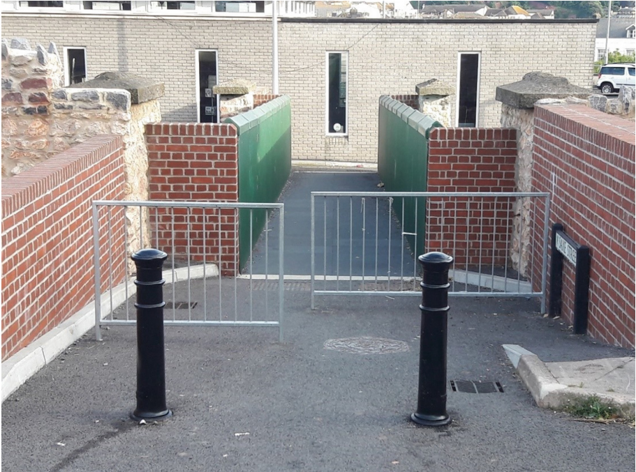
Fig. 4. View of the new FRP bridge including the new vehicle access restraint system, barriers and the resurfaced area.
