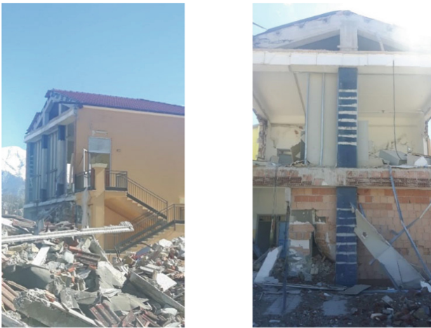
Fig. 1. Field survey after the Central Italy earthquake (2016).
