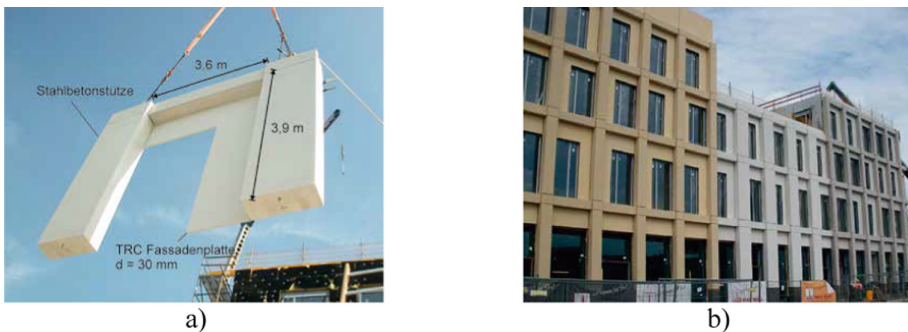
Fig. 1. Façade panel “Neuer Markt” a) During assembly, b) View of the completed façade panels (Image source: Firmengruppe Max Bögl).
