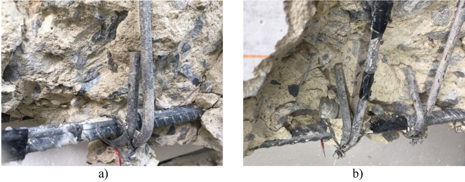
Fig. 10. Deformations of stirrups after removal of concrete covering a) 90° hooks [specimen B-90-150], b) and 135° hooks [specimen C-135-75].
