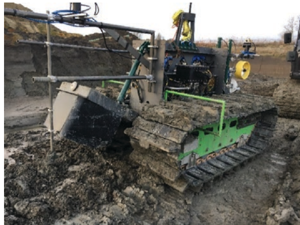
Fig. 6.5 Anchor for thrust–slip measurements (February 2017)
