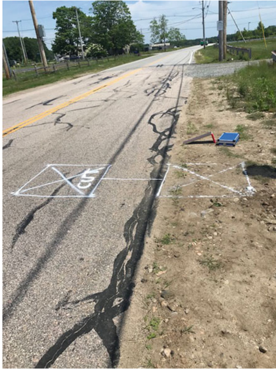
Fig. 7 Markings for the saw cuts for strain sensor (in the road) and energy harvester (in the shoulder) on Plains Road
