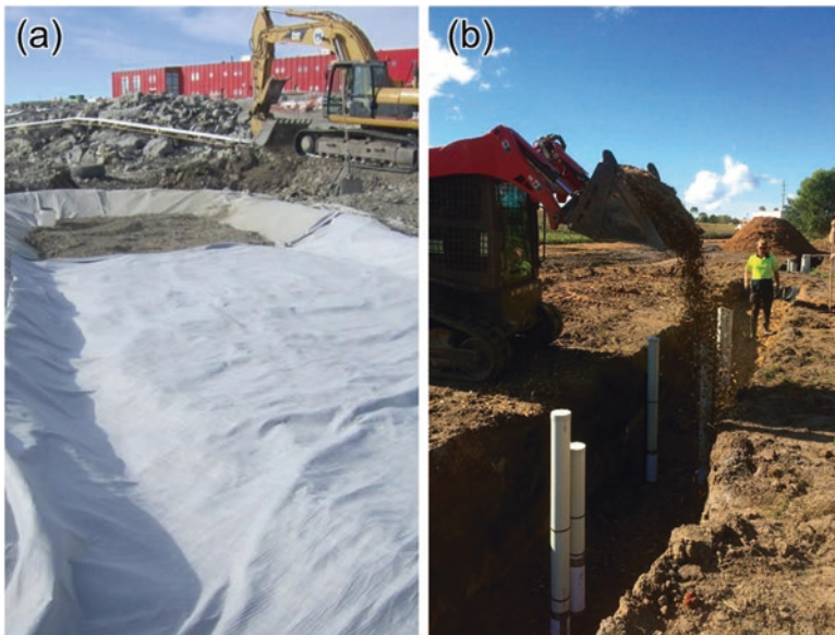
Fig. 11.12 (a) Hydrocarbon-contaminated soil being placed in a land-farming bioremediation cell lined with an impermeable geomembrane, Casey Station, Antarctica (used with permission from Australian Antarctic Division 2012); (b) bioreactor being constructed to promote denitrification for nitrate removal in SE Queensland, Australia. (From Wegscheidl et al. 2018 used under CC-BY-4.0)
