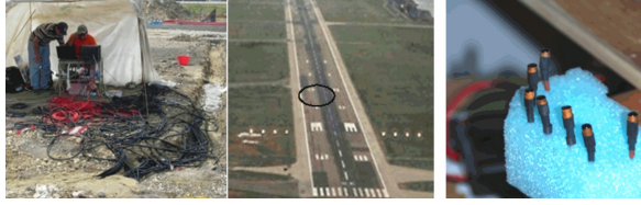
Fig. 4. Instrumentation installation at Italian SmartRunway at Cagliari airport
