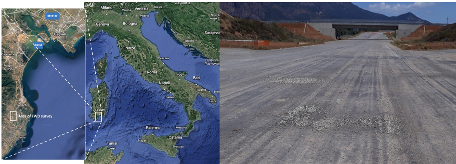
Fig. 1. Territorial context of SS195 road and its materials degraded due to action of atmospheric agents.
