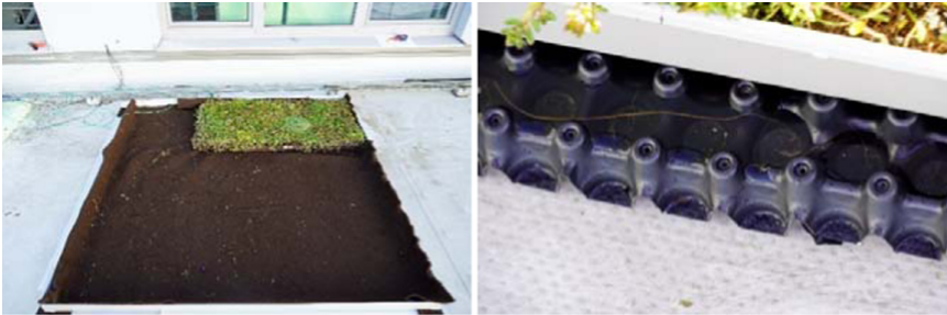
Fig. 5. Using of special boards from recycled waste and with already pre-grown vegetation. Right: drainage and retention layer.
