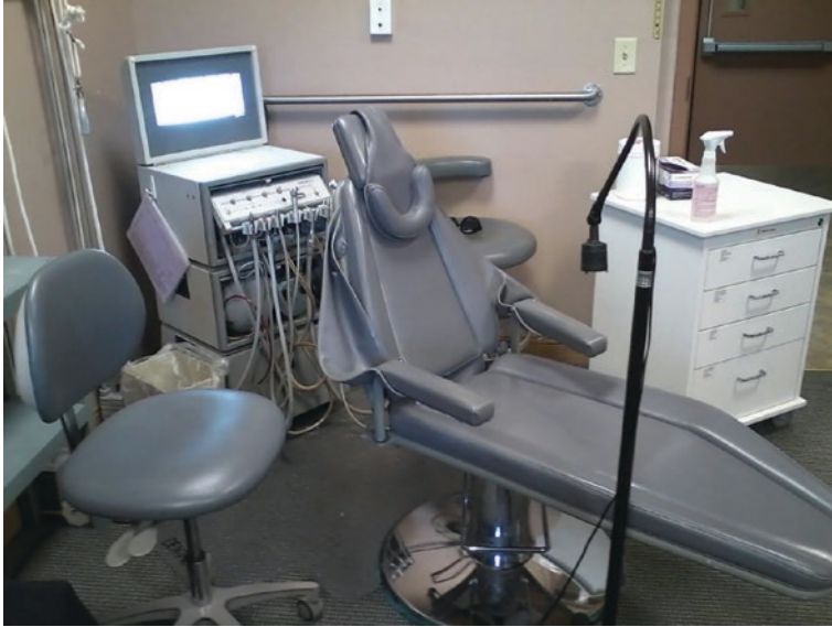
Fig. 6 An example of mobile equipment from DNTL (ProCart II) set up in a room in a nursing home with a portable chair and light, which is used by the University of Iowa's Geriatric Mobile Unit Program
