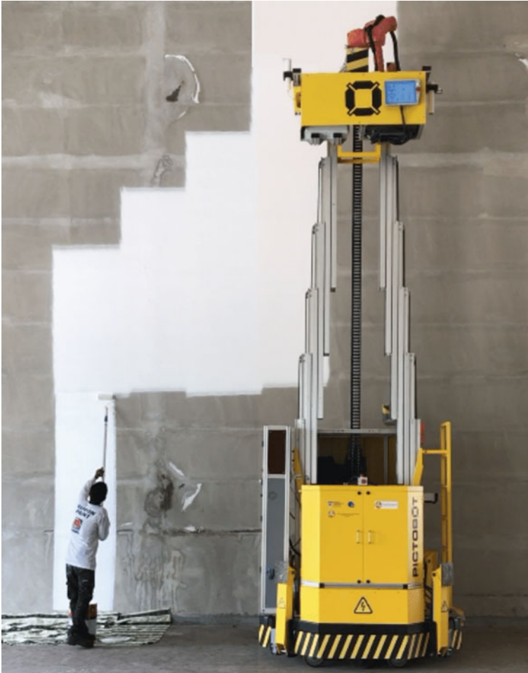
Fig. 7.17 PictoBot robot (automated spray painting of multiple vertical strips) (Asadi et al., 2018)
