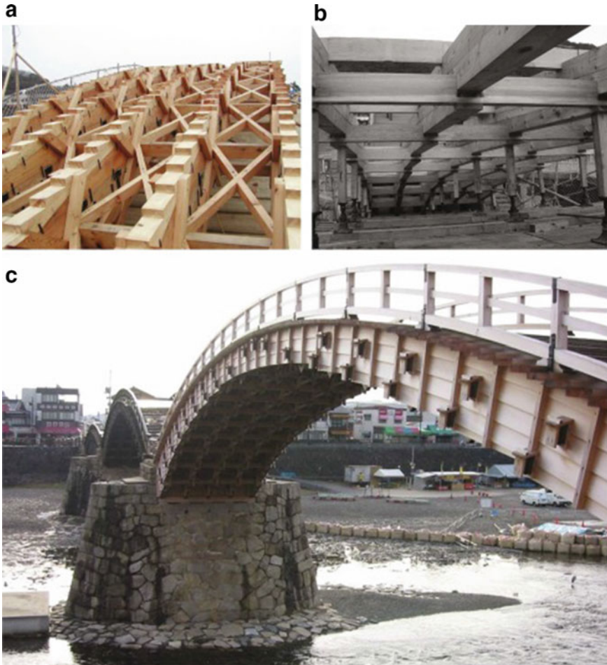
Fig. 5.14 Kintaikyo Bridge Reconstruction Project. a New arch ribs. b Falseworks for arch construction. c After replacement (Mohiuddin, 2015)
