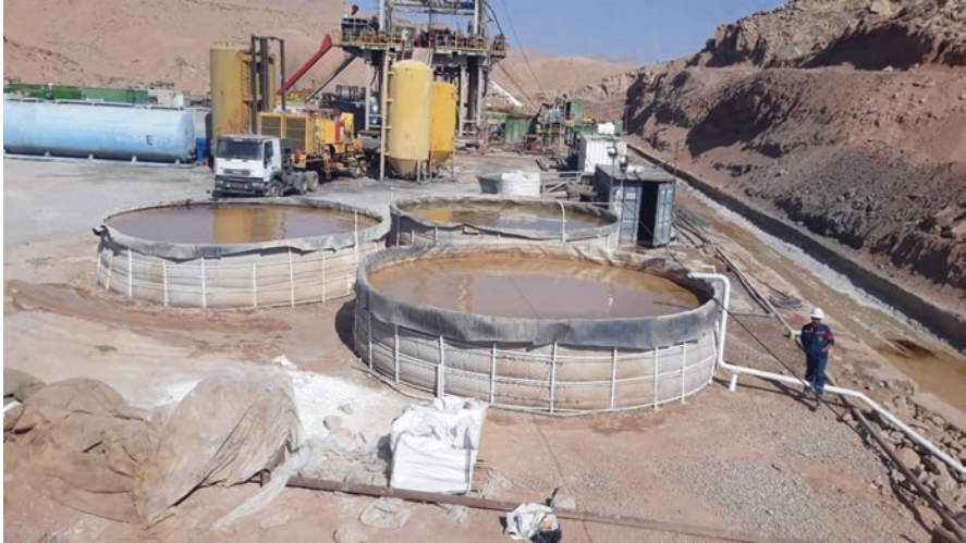
Fig. 4.4 Polyethylene cyclonic series of ponds mounted with iron structures. (Naft Sefid, Shushtar County, Khuzestan province, Iran, 2019)
