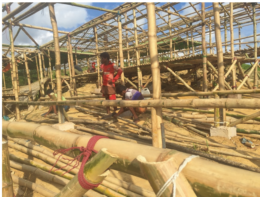
Fig. 7.5 Shelter construction and strengthening in camp. (Chakmakul camp, Cox's Bazar, Bangladesh, October 2018)
