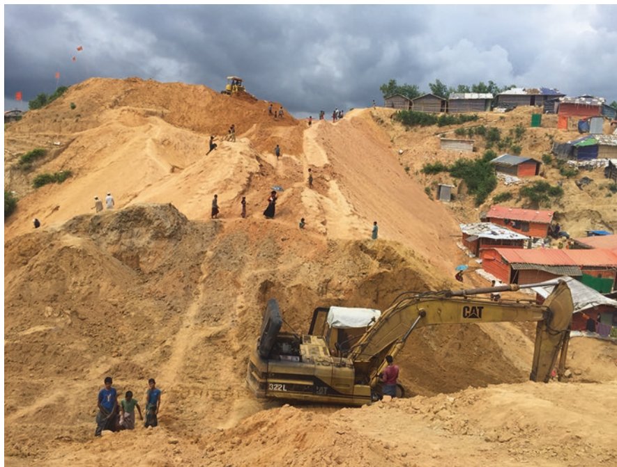
Fig. 7.4 Access road development in Rohingya refugee camps in Kutupalong-Balukhali, Cox's Bazar, Bangladesh, June 2018
