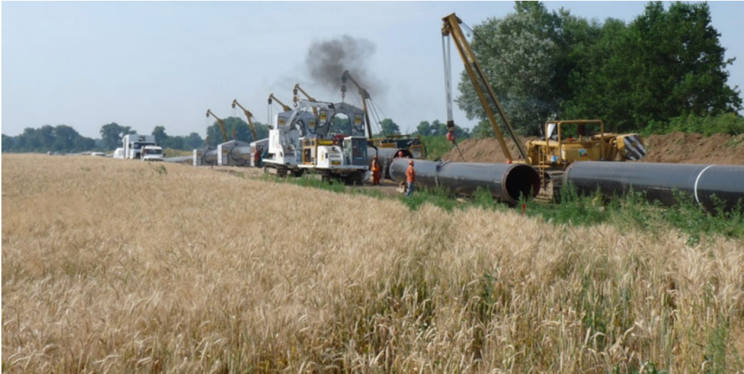
Fig. 2.7 Pipeline and cable laying for gas, power and communication lines causes physical disturbances of soil with long-term detrimental effects for soil health and plant rooting in many cases. Photo L. Mueller
