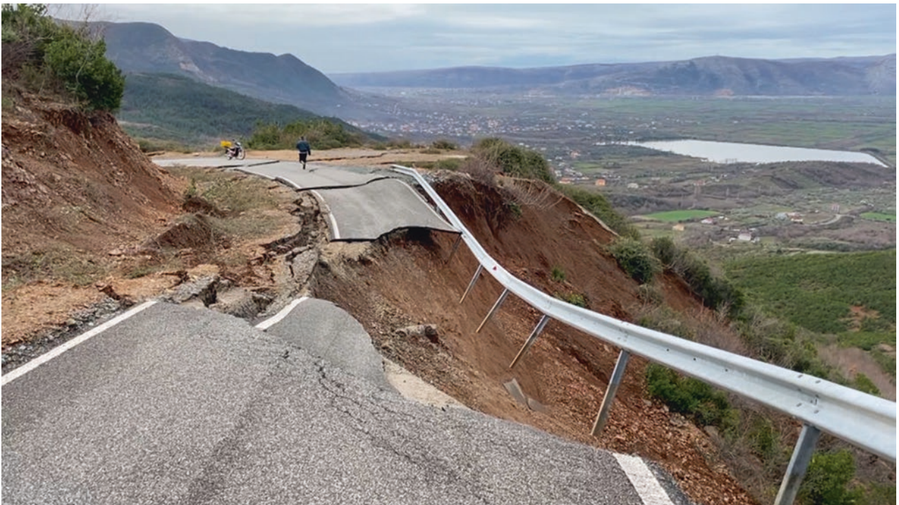
Photo 5.13 Destruction of the road by landslide (Qiriazı 2021)
