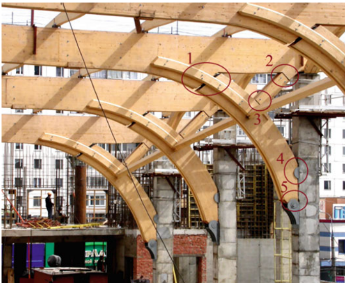
Fig. 2 Nodes of structures on glued-in rods that perceive compressive forces of the frame with a span of 36 m of training ice hall of the sports complex “Yantar” in Moscow
