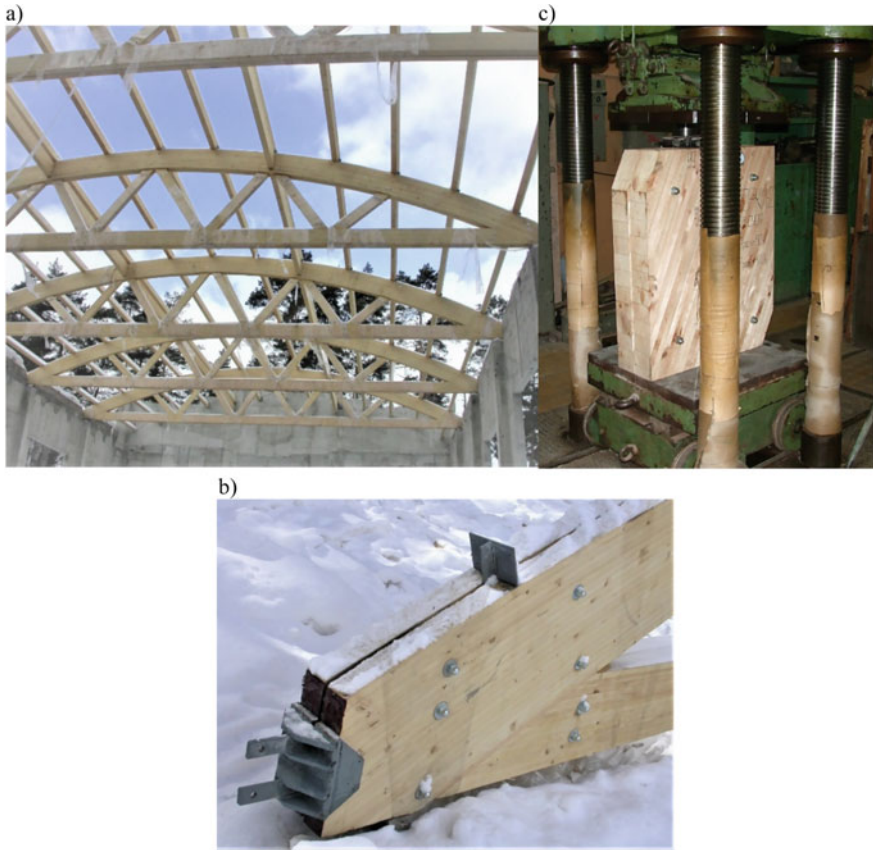
Fig. 3 Control tests of the fastening of the tightening in the support node of the truss covering the sports complexes in the village. Gorki-2, Moscow region: a general view of trusses in the process of installation; b support node; c fragment testing
