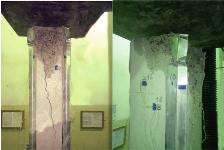
Fig. 12 Destruction of a steel–concrete rack
