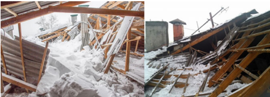
Fig. 2 Brittle destruction of the rafter system from the action of snow load (Russia, Udmurtia)
