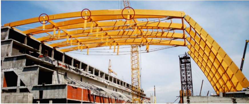
Fig. 1 Nodes of structures on glued-in rods that perceive compressive forces—the Aquatics Palace in Kazan with a crossbar in the form of a truss girder
