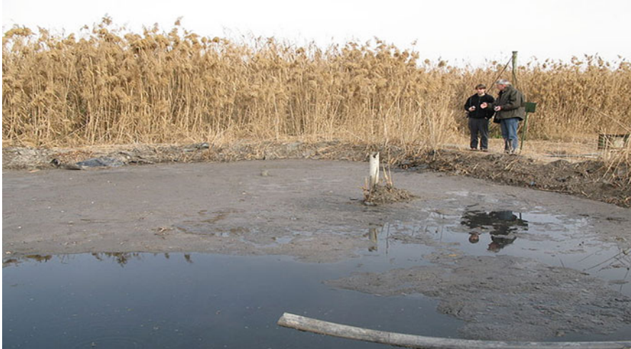
Fig. 3 Sludge drying bed
