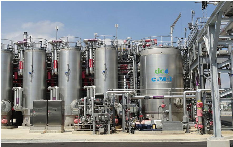
Fig. 1 Thermal hydrolysis system
