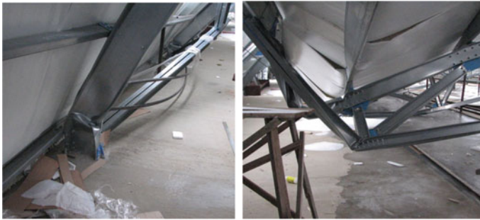
Fig. 2 Example of structures failures as local buckling of CFS members
