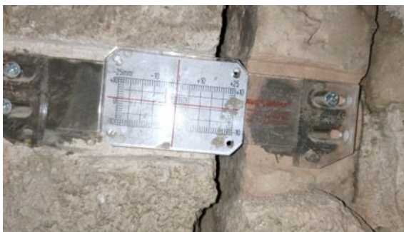
Fig. 4 Vertical crack with an opening width of at least 1 mm
