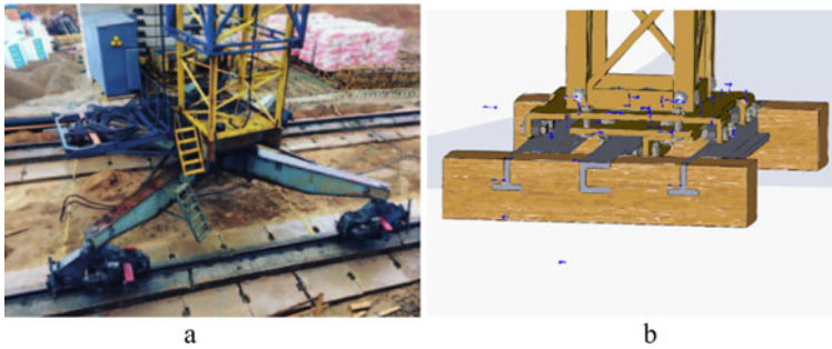
Fig. 5 Image of the base of a real tower crane (a) and its full-scale model (b)
