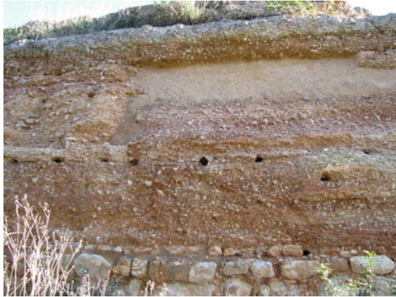
Fig. 6.5 Erosion at the base of a rammed earth wall in Paderne castle, Portugal
