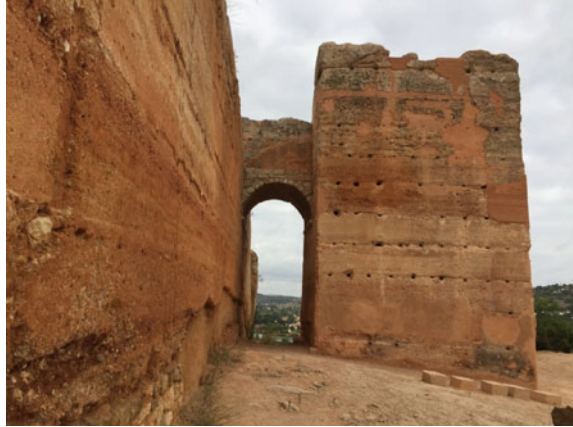
Fig. 6.2 Paderne castle in Algarve, Portugal, built in the twelfth century by using earth stabilised with air lime
