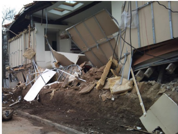
Fig. 6.1 Collapse of an earth building in Lyon, France, due to the accumulation of humidity at the wall base
