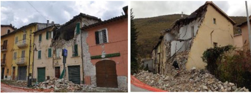
Fig. 2 Examples of local out-of-plane seismic damage to building aggregates, observed after the Central Italy sequence of 2016–2017 (Photos: A. Penna)
