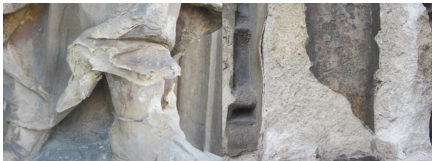
Fig. 4.3 Incompatible performance of treated limestone showing a thin hardened layer detaching from the powdery underlying stone. The strengthening of the consolidated layer was still effective, but its highly different physical properties led to a severe incompatible behaviour, ©José Delgado Rodrigues
