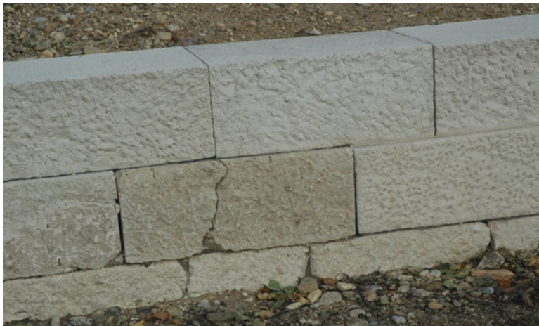
Fig. 7.8 A large artificial stone with severe cracking after 2 years from its manufacture
