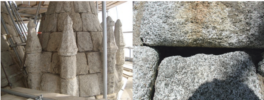
Fig. 4.6 Lantern of Evora Cathedral. Sand disintegration of granite and extensive deterioration of joints were the main problems to address, ©José Delgado Rodrigues
