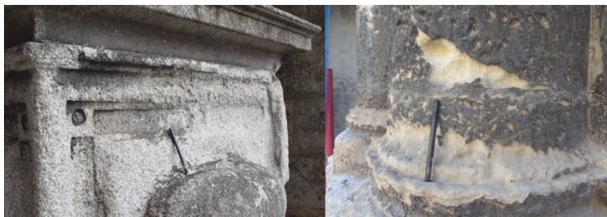
Fig. 4.2 Significant mass losses can occur in localised areas that require consolidation, and the approach to follow is primarily specific to each situation. Examples of granular disintegration in granite from S. Francisco church (Porto, Portugal), and powdering in a soft limestone from Avignon (France), ©José Delgado Rodrigues
