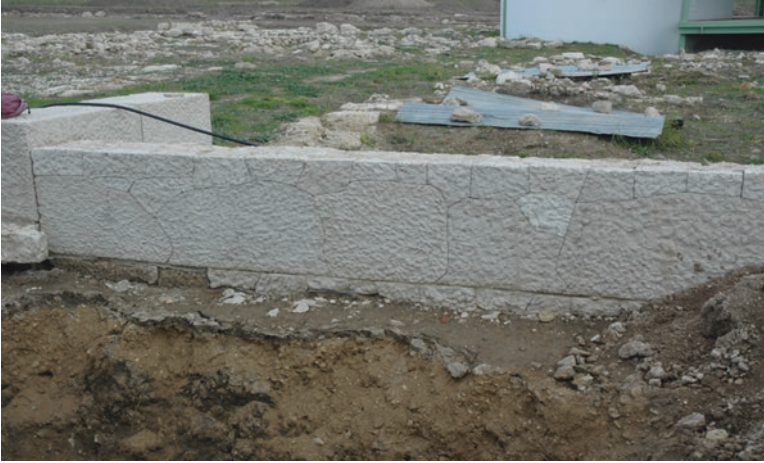
Fig. 7.9 Thin cracks in the new artificial stone
