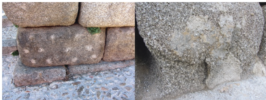
Fig. 4.7 Segovia Aqueduct (Spain). The deep injection of epoxy resins in a fairly sound block (left) was useless, while the similar injection in the heavily decayed block (right) has left the surface unconsolidated and subject to active sand disintegration and significant mass loss, ©José Delgado Rodrigues
