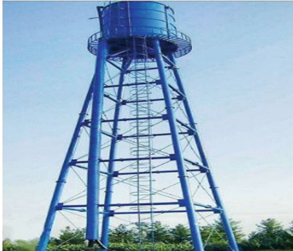
Fig. 12.4 Image of elevated water tank
